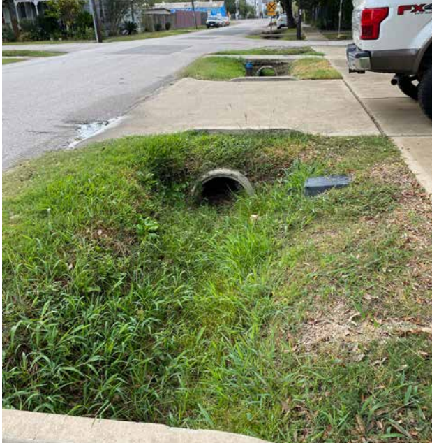
Open Ditch Drainage Presents Challenges
